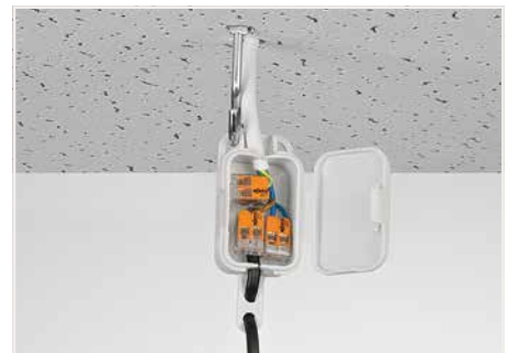
Pendant light connection in suspended ceilings
