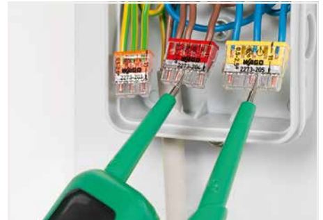
Testing via test port opposite to conductor entry.
