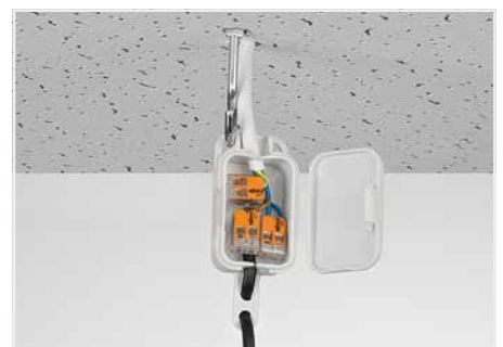
Pendant light connection in suspended ceilings
