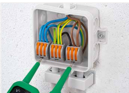
Testing the wired connectors.
