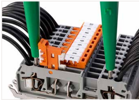
Testing with voltage tester.
