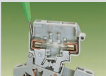
Voltage test, either at input or output with fuse holder in closed position (live)
