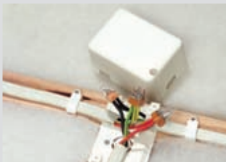
Push-wire connectors used in a junction box. (Australia)
