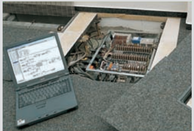
Floor distribution boxes
