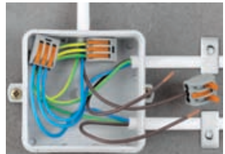
Wiring of flexible conductors in a junction box
