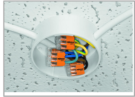
Lighting distribution in ceiling canopy
