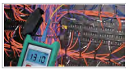
Fiber optic power test
