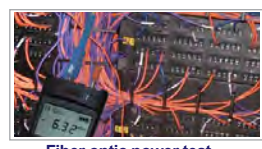
Fiber optic power test
