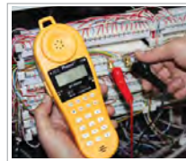
Telephone line testing
