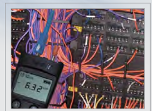
Fiber optical power test
