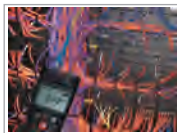
Fiber optic power test
