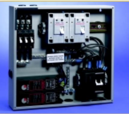
Power distribution center with ground fault circuit protectors and various breakers
