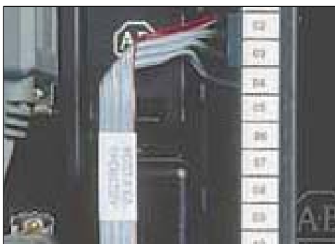
Terminal Block Labeling
