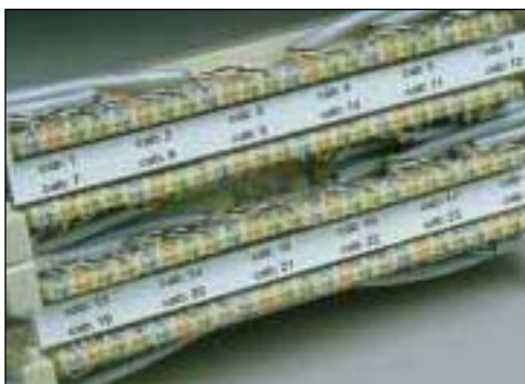
Network Systems Labeling
