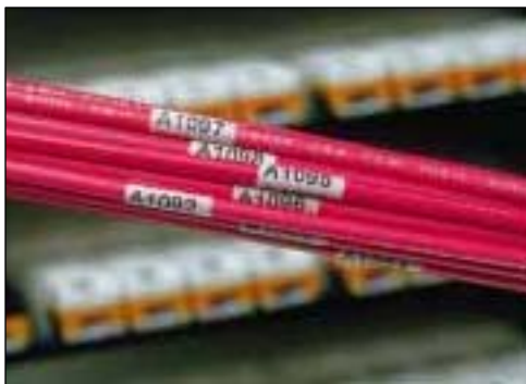
Wire and Cable Identification
