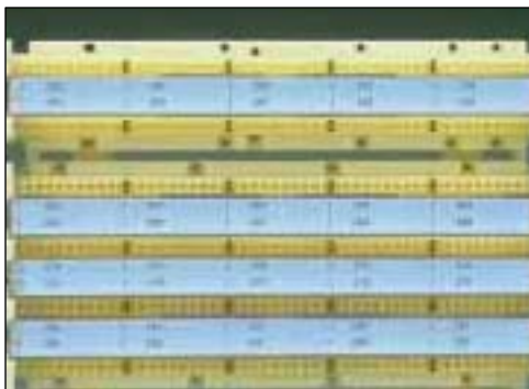
Network Systems Labeling
